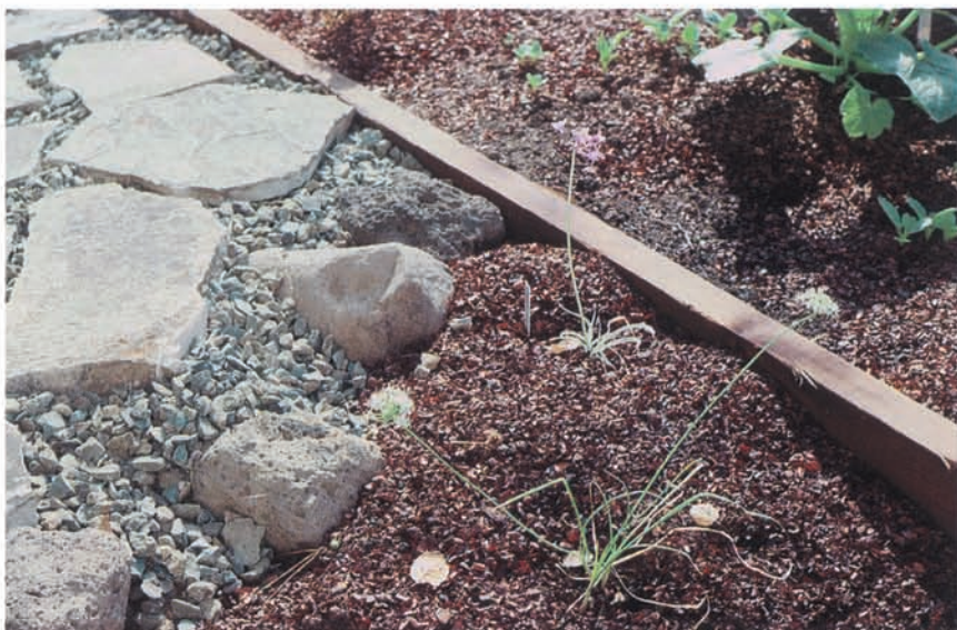
Figure 1.14 Flagstones are set in packed gravel, without a plastic undersheet, for good percolation of winter rain. The stones' pleasing texture makes a safe, all-weather surface.
